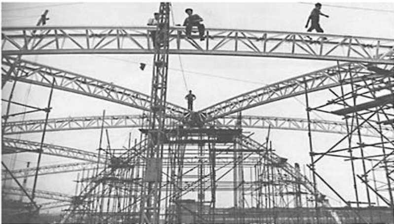
Alloy girders support the framework of the Dome of Discovery, for the 1951 Festival of Britain. (Photograph taken July 1950.)
