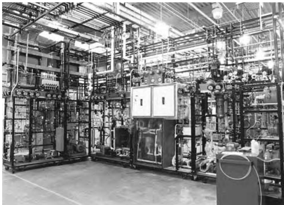
Fig. 3 An integrated pilot plant installed in an open bay. (View this art in color at www.dekker.com .)
