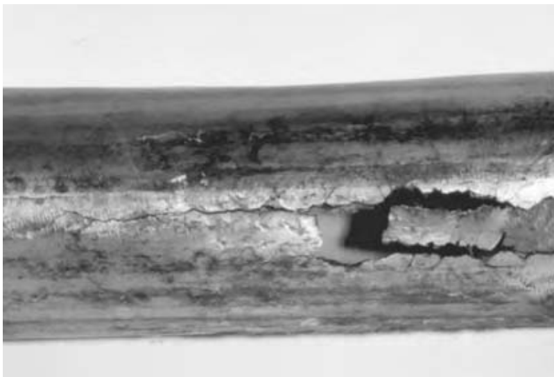
Fig. 5 External SCC of a stainless steel pipe after contact with wet, chloride-containing, thermal insulation.
