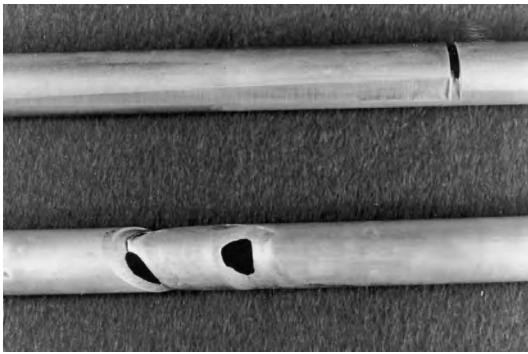
Fig. 2. Heat exchanger tubes cut through at supports and damaged by impacting from broken tubes due to flow-induced vibration.
