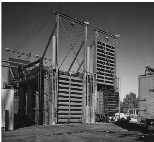
Fig. 15. Vacuum cooler of railroad-car size. (Gay Engineering Corp.)
