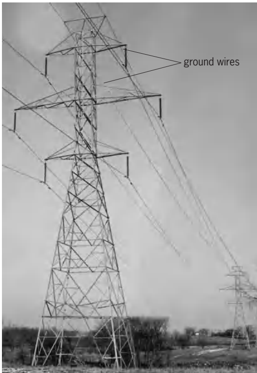
Fig. 3. Double-circuit suspension tower on the Olive-Gooding Grove 345-kV transmission line, with two circuits strung and with two ground wires. (Indiana and Michigan Electric Co., American Electric Power Co.)
