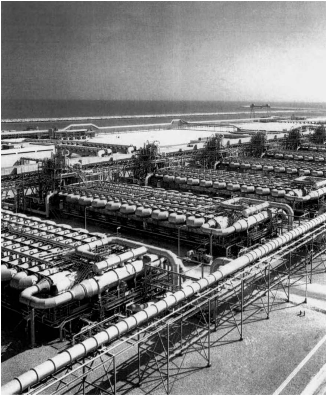
FIGURE 1 Panoramic view of the Al-Jubail Saudi Arabia, phase II, MSF desalination plant. It is up to now the World largest desalination installation totaling a capacity of 947,000 m 3 /d (250 Mgd) fresh water production. Each unit has a capacity of 23,500 m 3 /d (6.2 Mgd). The plant was built for the Saline Water Conversion Corporation, of Saudi Arabia by the Japanese Companies of Sasakura and Mitsubishi. (Courtesy Sasakura Engineering Co., Japan)
