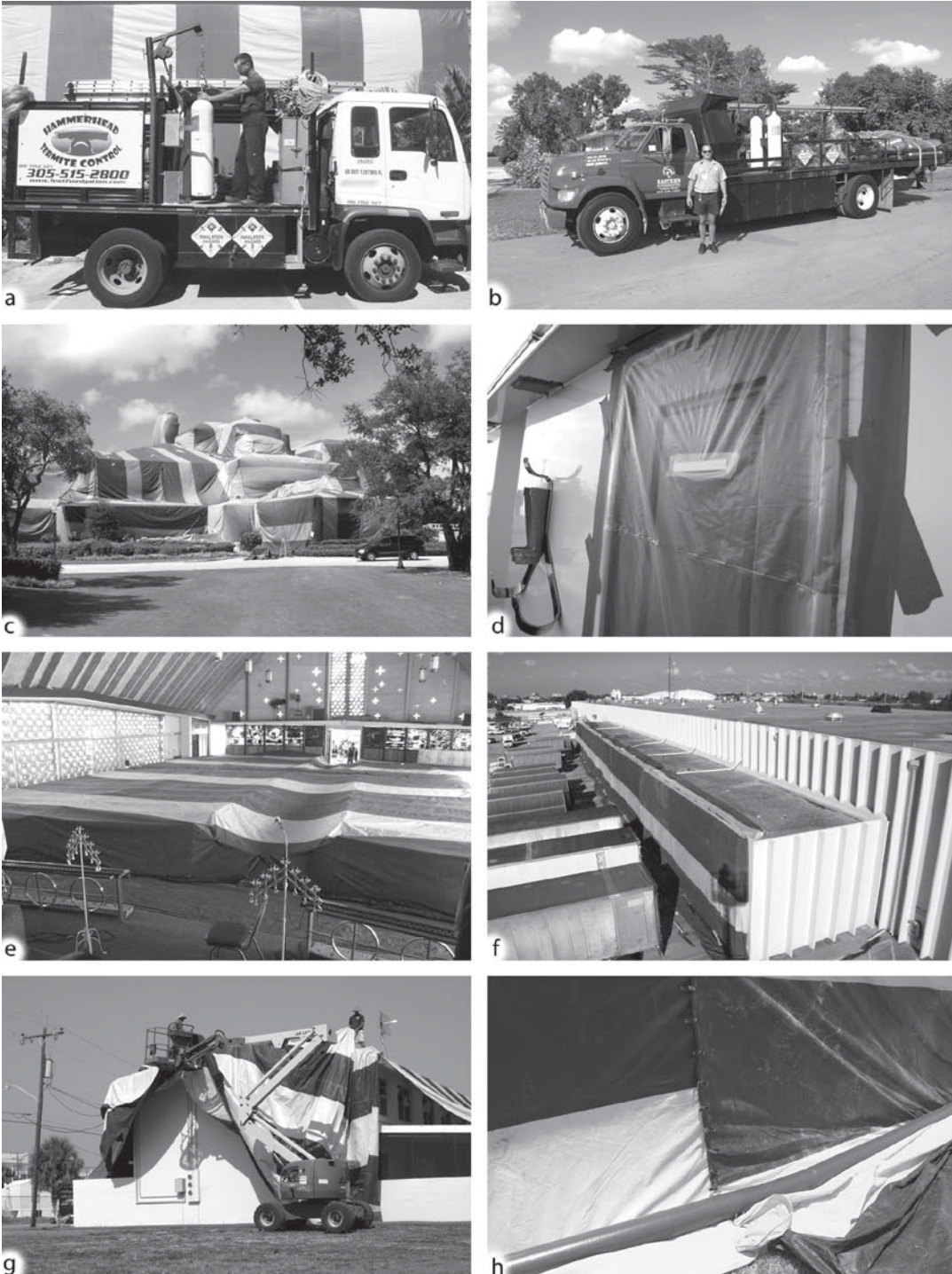
Structural Fumigation, Figure 145 Fumigation of structures: (a) a compact truck for narrow streets, (b) a full size truck provisioned to transport equipment, chemicals, and crew members to a fumigation site, (c) tarpaulin fumigation of a mansion, (d) “tape and seal” fumigation of a boat (exterior door shown), (e) compartmental fumigation of church pews, (f) a combination tarpaulin and “tape and seal” fumigation of a warehouse (g) mechanical lift to raise tarpaulins onto building, (h) water “snake” for proper ground seal.
