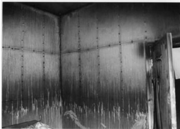
Figure 4 Smoke tends to deposit preferentially on cooler surfaces and may reveal positions of nails and joints normally hidden by the plaster.
