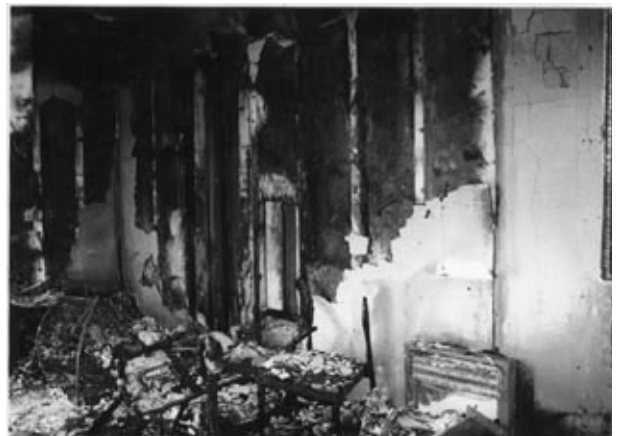
Figure 2 A characteristic funnel pattern indicating an armchair as the point of ignition. The fire had, in fact, been ignited approximately 500 mm from the chair, but had spread to it at an early stage in the fire.
