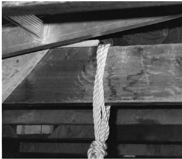
Figure 1 Photograph showing multiple grooves worn into the beam with rope in situ. Demonstrates evidence of prior autoerotic activity of a similar nature.
