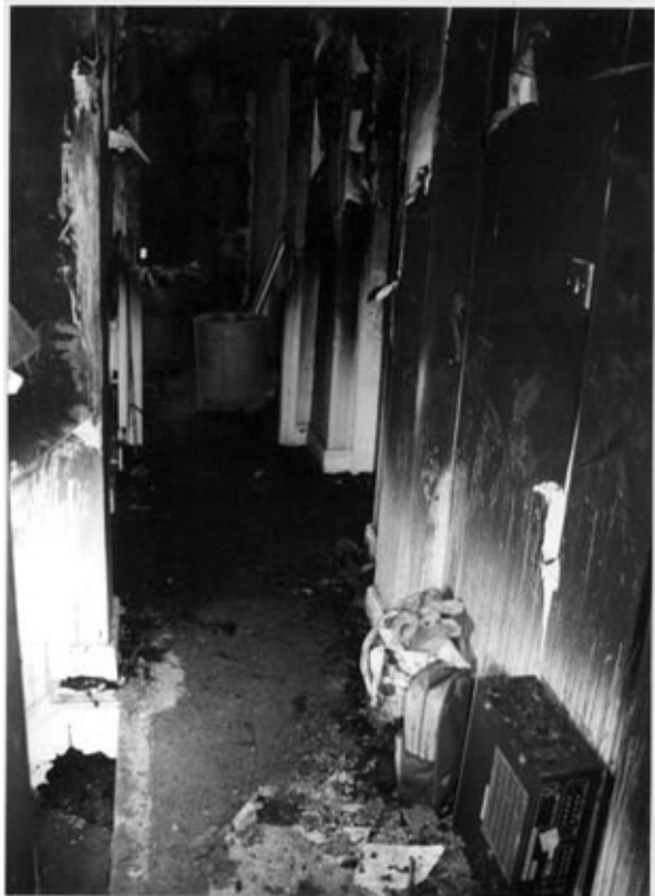
Figure 3 Typical smoke-logging in a passageway. Hot, buoyant smoke produces staining at a high level.
