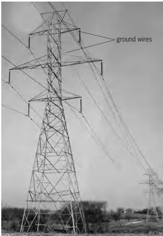
Fig. 3. Double-circuit suspension tower on the Olive-Gooding Grove 345-kV transmission line, with two circuits strung and with two ground wires. (Indiana and Michigan Electric Co., American Electric Power Co.)
