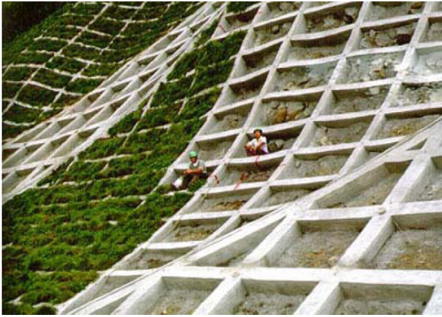
Figure A26 Road construction in Hokkaido, Japan. Much effort is made to stabilize the slopes, but landslides are common in Andosol areas.
