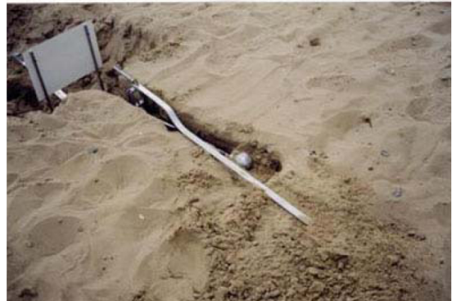
Figure S43 A schematic view (upper) and field installation (lower) of the measuring system for soil stress and deformation determination.
