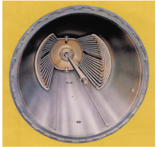
Fig. 2: Steam/water heat exchanger tubes in a beam dyeing machine (Platt Longlose).
