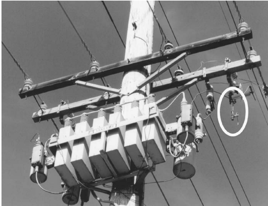
FIGURE 6.14 Capacitor bank with a blown fuse. (Copyright © 2002. Electric Power Research Institute. 1001691. Improved Reliability of Switched Capacitor Banks and Capacitor Technology . Reprinted with permission.)
