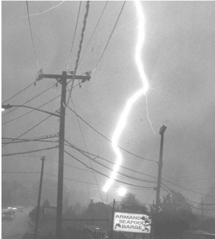
FIGURE 12.28 Lightning-caused fault on a Long Island Lighting Company 13-kV circuit. (From Short, T. A. and Ammon, R. H., "Monitoring Results of the Effectiveness of Surge Arrester Spacings on Distribution Line Protection," IEEE Trans. Power Delivery , 14(3), 1142-1150, July 1999. ©1999 IEEE. With permission.)
