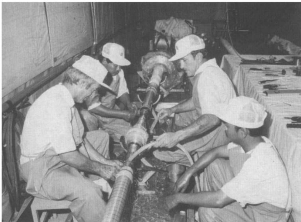
Fig. 35.18 Joint bay with 275 kV stop joint for fluid-filled cable
