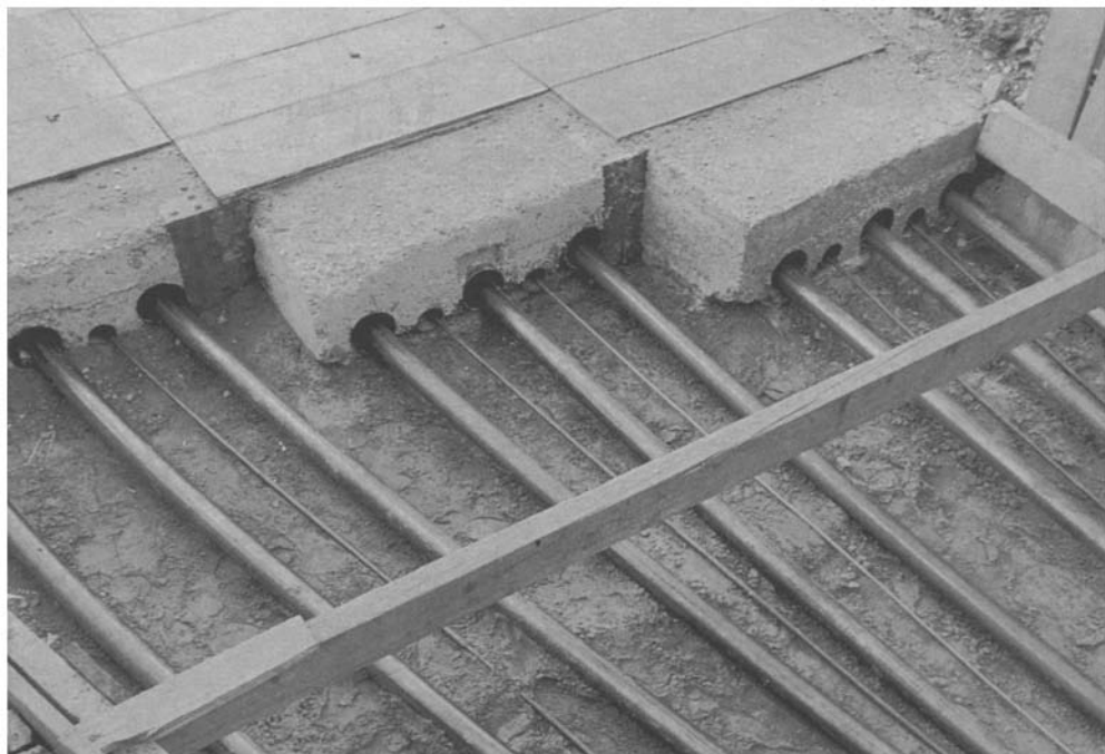
Fig. 36.1 A triple circuit of 132 kV XLPE insulated cables installed in a duct block
