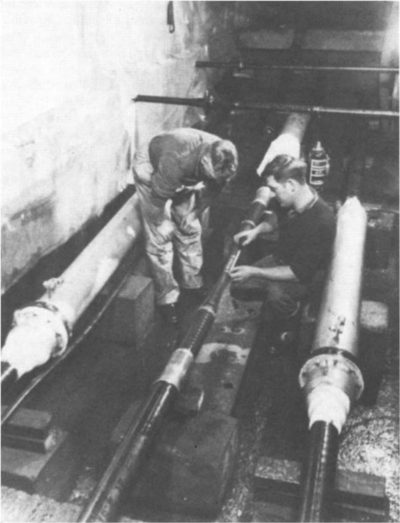
Fig. 35.17 Joint bay for 275 kV fluid-filled cables
