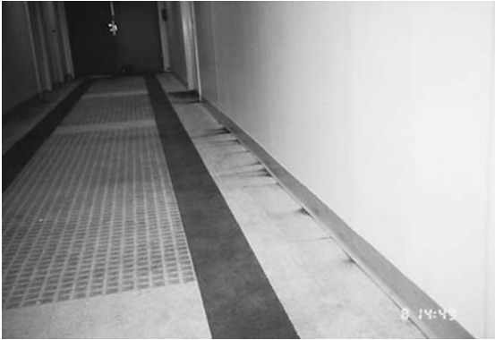
FIGURE 7.2 An Explosion is a Fire that Occurs in Milliseconds. Here Soot Was Deposited on the 97th Floor by the Supersonic Forces Generated.
