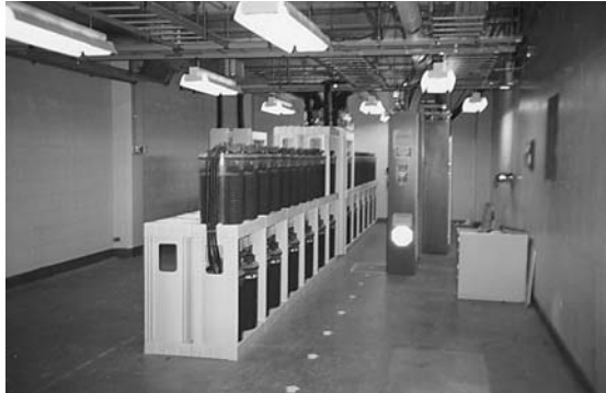
FIGURE 7.5 Batteries for UPSs and Office Power Should Be Isolated from the Rest of the Electronic Equipment to Prevent Corrosion from a Faulty Battery's Emissions.
