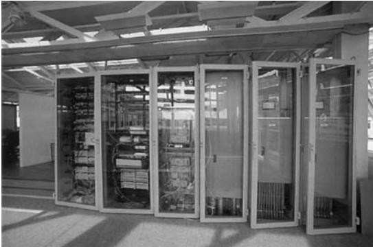
FIGURE 12.22 The Intelligent Workplace Demonstrates Distributed Satellite Closets Which Are Modular and Relocatable, Customized for Working Neighborhoods of 35–50 People, with Modular Racks Supporting Fiber, Data, and Voice Patch-Panels, Routers, Servers, Environmental Control and Security Modules. While Most 10,000 ft 2 Neighborhoods Might Need Two Modular Closets, This Laboratory Demonstrates Extensive Power Submetering and Competitive Control Systems Requiring Six Closets.
