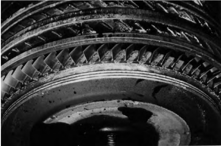
Figure 13-7. View of last stage compressor blades with contamination evident on and between blades. 5,000 horsepower gas turbine-generator unit after 44,500 hours operation.
