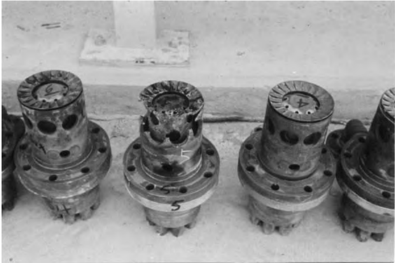
Figure 13-13. Burnt fuel nozzles from can-annular combustor. 55,000 horsepower gas turbine-generator with less than 10,000 operating hours.
