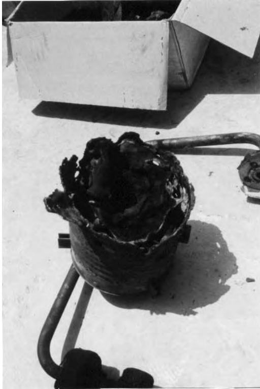
Figure 13-9. Can-annular combustor failure due to liquid carry-over in the fuel gas. 30,000 horsepower gas turbine-pump drive unit with less than 24,000 operating hours.
