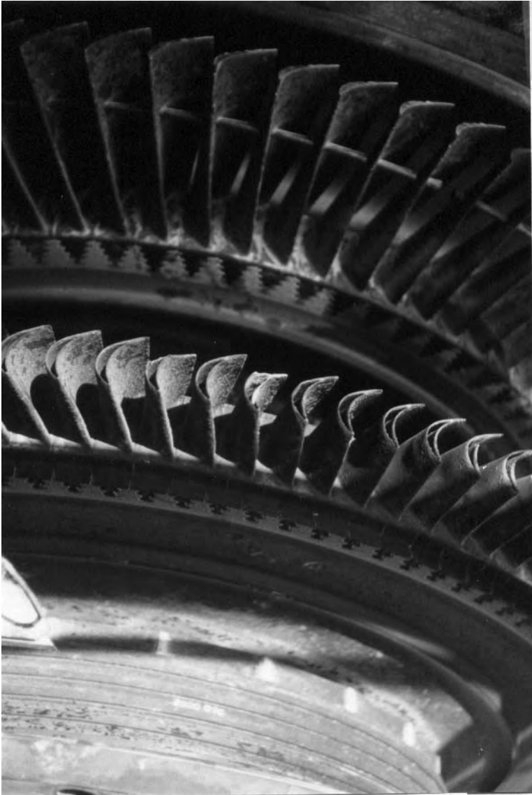
Figure 3-7. Courtesy of Power & Compression Systems. This is a 1970 vintage gas turbine designed with lacing wire to dampen the second stage turbine blades. Note the hollow 1st stage turbine blade indicating blade cooling and the corrosion on both the 1st and the 2nd-stage blades.
