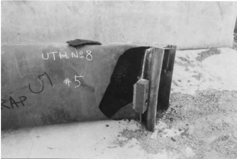
Figure 13-11. Can-annular combustor transition piece failure due to brittle fatigue due to fretting. 55,000 horsepower gas turbine-generator with less than 10,000 hours operation.
