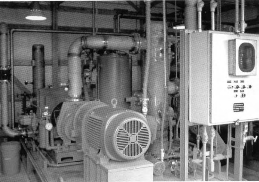
Figure 17-4. Gas Compression System
