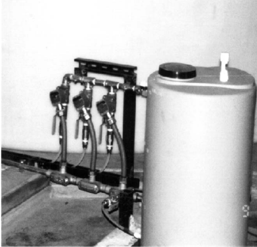
Figure 50 Biocide injection tank with distribution manifold. The metering pumps are not shown on the picture.
