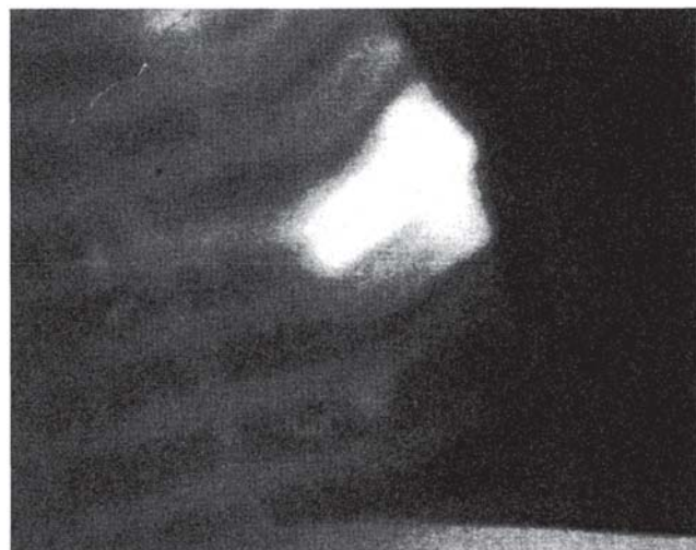
Figure 14.25 Thermal hot spot near the end of the stator core. (Courtesy of the Ohio Edison Company, Akron, Ohio.)
