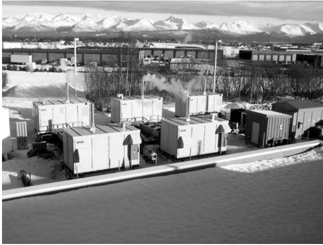
FIGURE 8.9 Five PC25 power plants provide primary power for a major postal sorting facility in Anchorage, AK. Since beginning operations in 2000, the units have ensured that the facility has never lost power, despite numerous grid disturbances. (Photograph courtesy of UTC Fuel Cells.) (Please check Color Figure 8.10 following page 9-10.)
