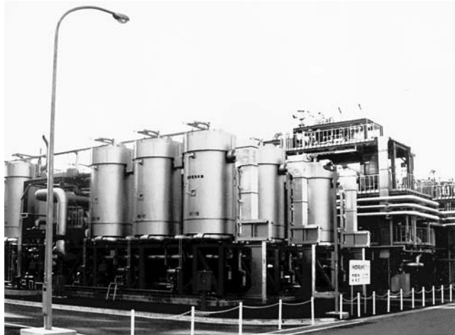
FIGURE 2.16 The 11-MW plant in Goi, Japan based on PC-23. The fuel cells are contained in the upright cylindrical vessels. (Courtesy of UTC Fuel Cells.)
