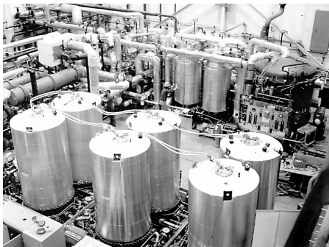
FIGURE 2.15 The PC-19 1-MW plant, with the phosphoric acid fuel cells contained in the upright vessels. Carbon was used as support for the fuel cell catalysts, reducing the platinum loading. (Courtesy of UTC Fuel Cells.)
