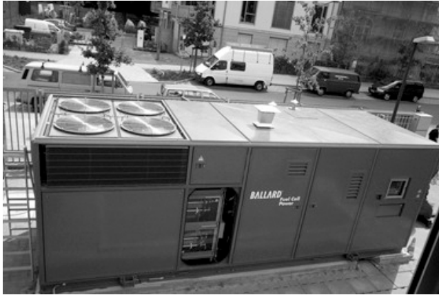
FIGURE 8.7 The 250-kW Ballard Generation Systems PEMFC power plant installed in Berlin in 2000. (Photograph courtesy of Ballard Power Systems.) (Please check Color Figure 8.7 following page 9-10.)
