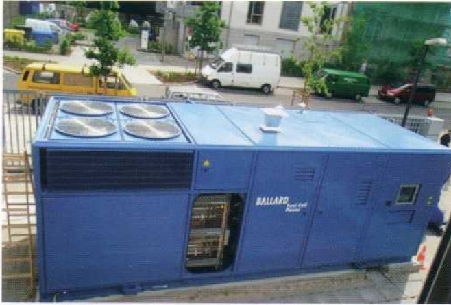
CHAPTER 8, COLOR FIGURE 8.7 The 250-kW Ballard Generation Systems PEMFC power plant installed in Berlin in 2000. (Photograph courtesy of Ballard Power Systems.)
