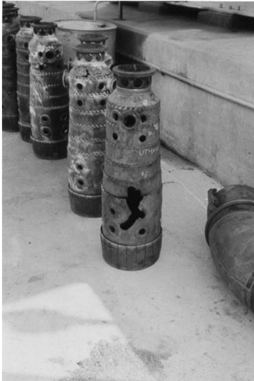
Figure 13-10. Can-annular combustor failure (burning and cracking) due to liquid mist in the fuel gas. 55,000 horsepower gas turbine-generator unit with less than 10,000 operating hours.
