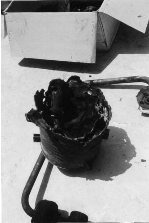
Figure 13-9. Can-annular combustor failure due to liquid carry-over in the fuel gas. 30,000 horsepower gas turbine-pump drive unit with less than 24,000 operating hours.
