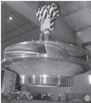
(a) Water TG unit for high-head pumped, storage power station (360 MW, 50 Hz, 12 poles, 500 rpm)
