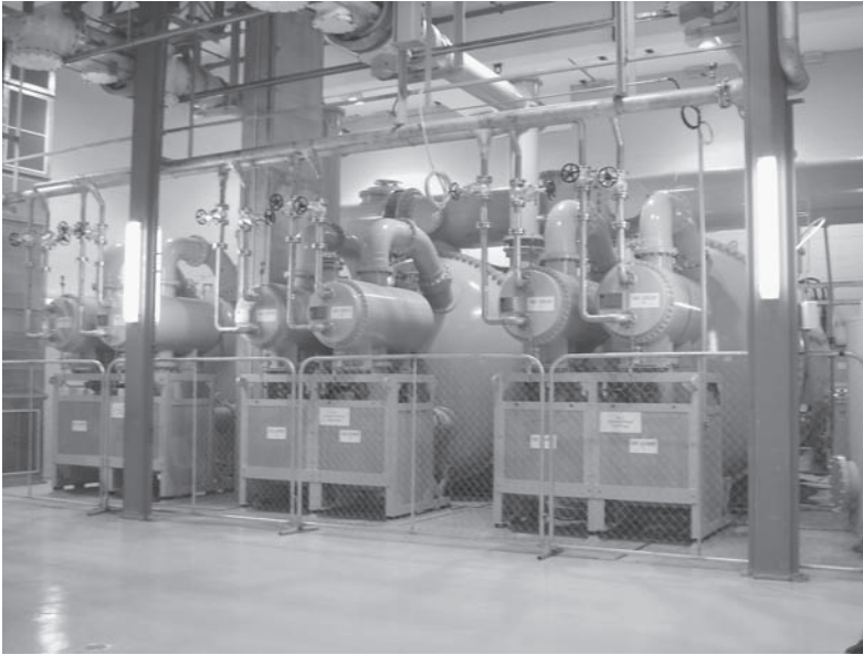
Haymarket substation (Australia)
