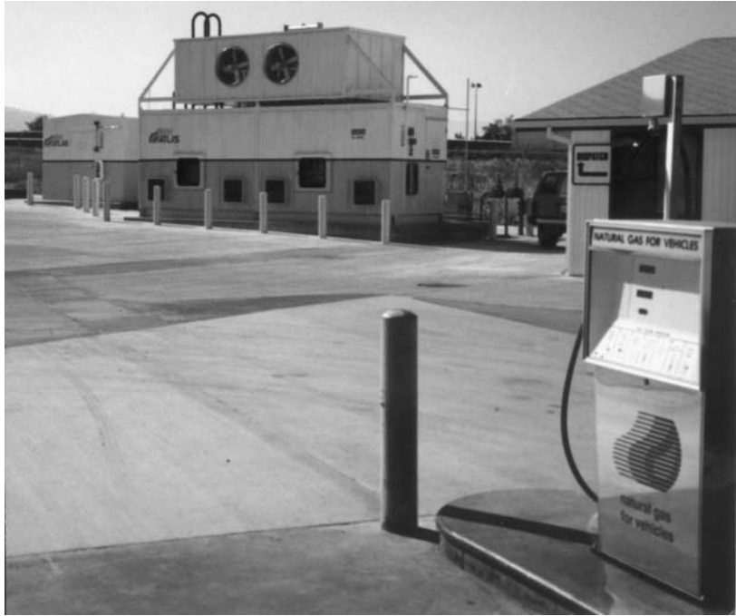
FIGURE 8.1 Compressed natural gas refueling station (courtesy of IMW Altas Inc.).
