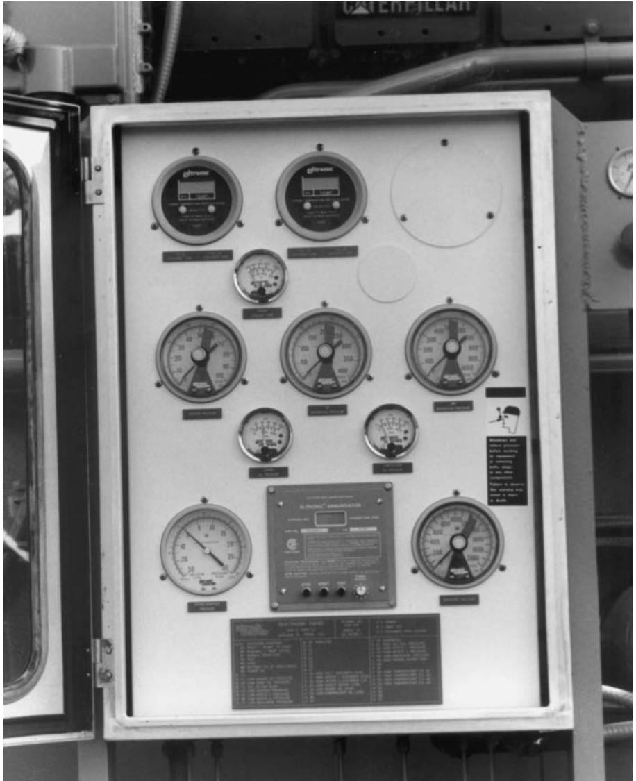
FIGURE 23.8 Typical electric panel.
