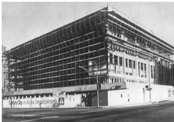
FIGURE 5.9 This shows Tubelox scaffolding used to scaffold building surfaces with a difficult roof-overhang condition. The versatility of Tubelox is similarly utilized for cooling towers, spheres, and refinery structures.
