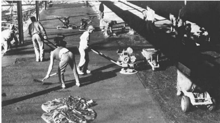
FIGURE 2.2 The application of a separate \frac{3}{4} -in. low water-cement ratio floor topping to a previously placed concrete base slab produces a wearing surface that is denser and more wear resistant than monolithically placed floors.
