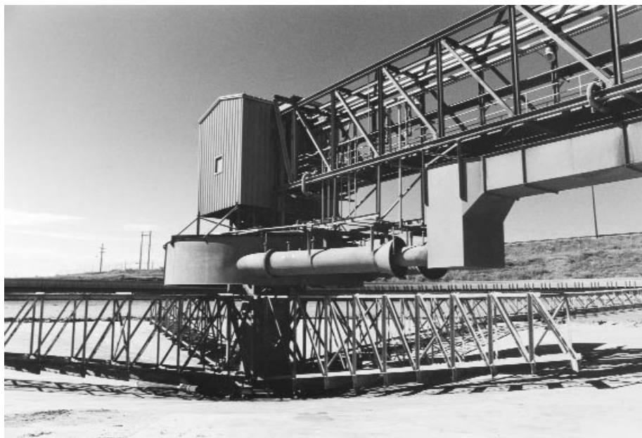
FIG. 18-92 E-Duc® Feed dilution system installed on 122-m-diameter thickener. (EIMCO Process Equipment Co.)
