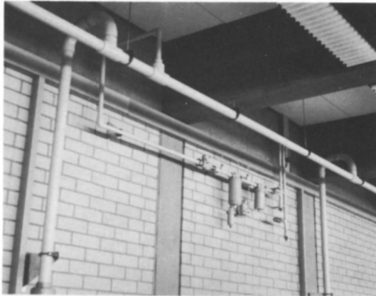
FIGURE 2 – ABS air line installation. ( Durapipe – S+LP, Glynwed Pipe Systems )
