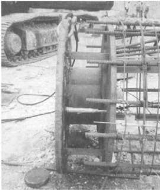
FIGURE 9.32 Osterberg cell being set up for load testing. (Courtesy of LoadTest, Inc. www.loadtest.com .)
