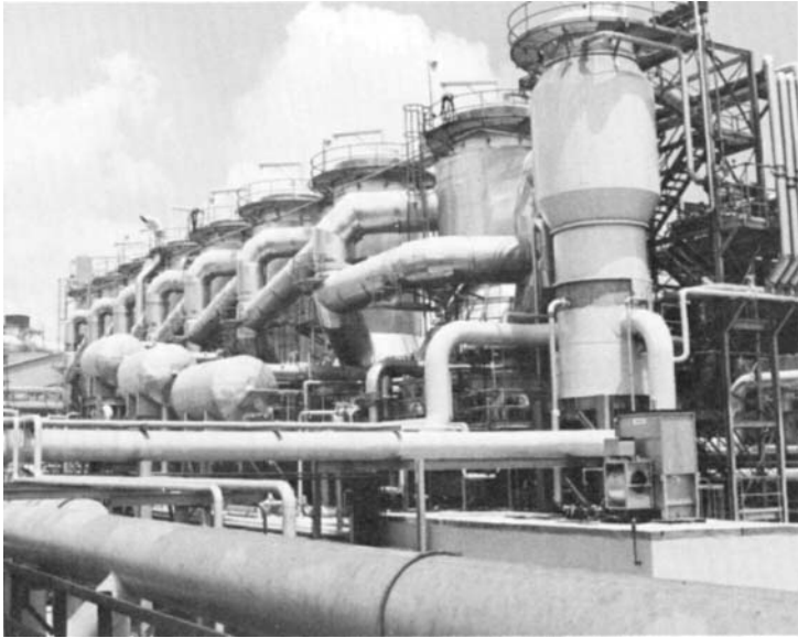
FIG. 18.6 Black liquor evaporator in a kraft pulp mill. Some of the condensate may be recovered for reuse, but much of it is contaminated with sulfur compounds. (Courtesy of HPD Corporation.)
