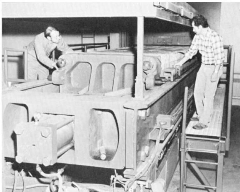
FIG. 9.48 A plate-and-filter press dewatering sewage plant sludge conditioned with polymer. Polymer increased throughput and eliminated 400 lb per ton inorganic ash previously produced by lime/ferric chloride treatment.
