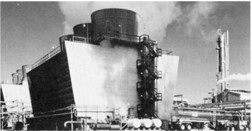
FIG. 38.12 Induced-draft tower. Air enters the tower louvers and is well distributed before exiting at top.
