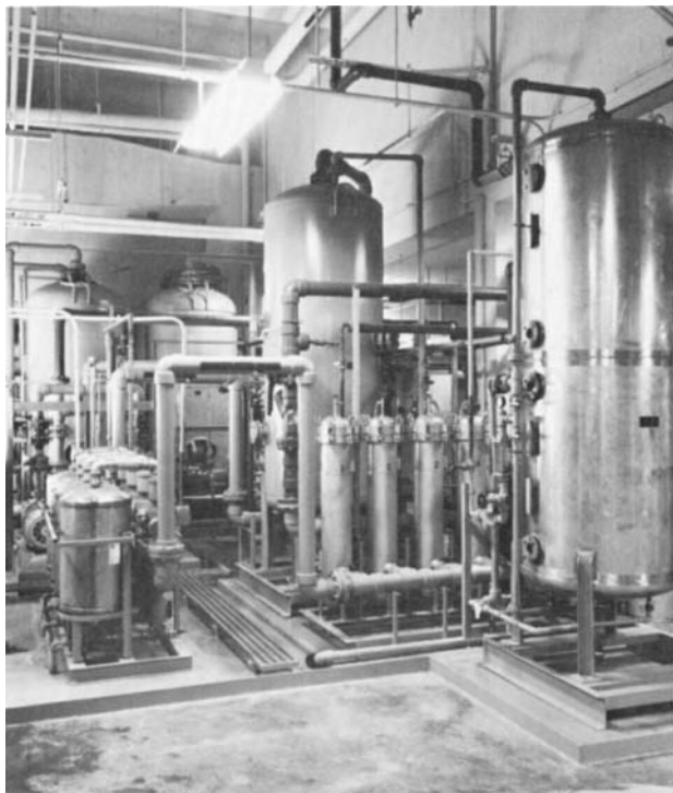
FIG. 15.1 Ultrapure water is needed in many areas of manufacture of electronic components. The final step in the treatment system shown here is membrane filtration following several stages of ion exchange. (Courtesy of Bell Laboratories.)
