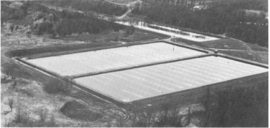
FIG. 23.7 An aerated facultative lagoon for treatment of sewage from a community of approximately 5000 people. (Courtesy of Hinde Engineering Company.)
