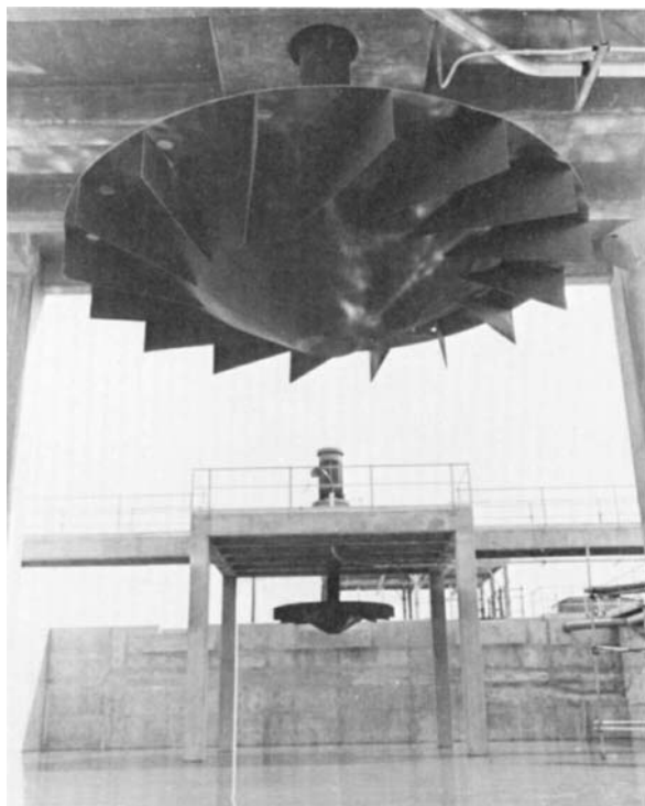
FIG. 16.3 Details of construction of a fixed-position surface aerator, shaped to produce high-volume pumping and air entrainment. (Courtesy of Infilco Degremont Inc.)
