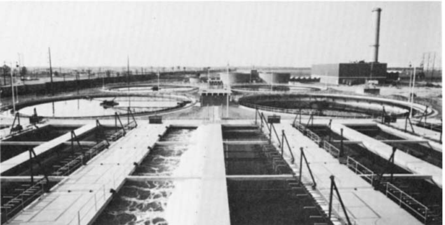
FIG. 16.2 Air diffusers in municipal sewage treatment plant. The diffuser assemblies may be retracted, as in basin on right, for maintenance and to prevent clogging when basin is out of service. (Courtesy of FMC Corporation.)
