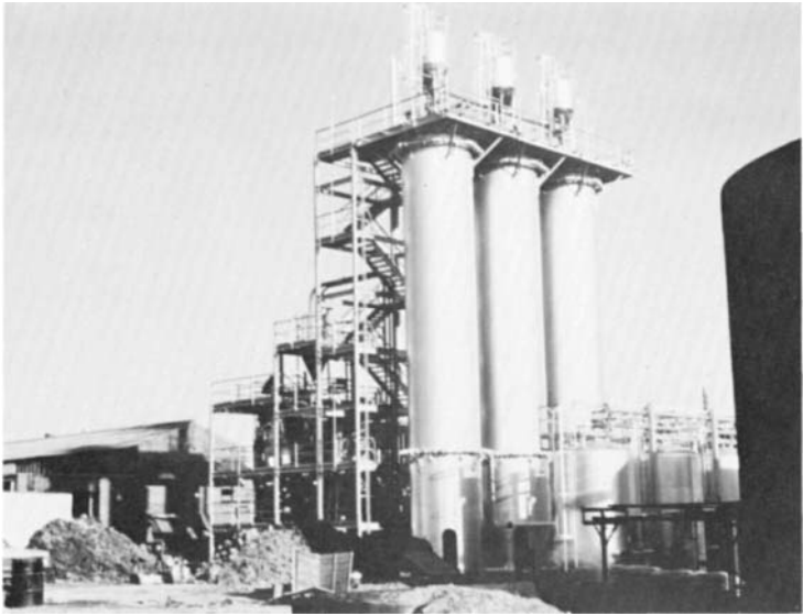
FIG. 17.10 A 2000 gal/min countercurrent activated carbon system treating refinery wastewater. Each column is 10 ft 0 in in diameter with an overall height of 65 ft 0 in and bed depth of 45 ft 0 in. A 5 ft 0 in diameter multiple hearth furnace regenerates spent carbon. (Courtesy of Illinois Water Treatment Company.)
