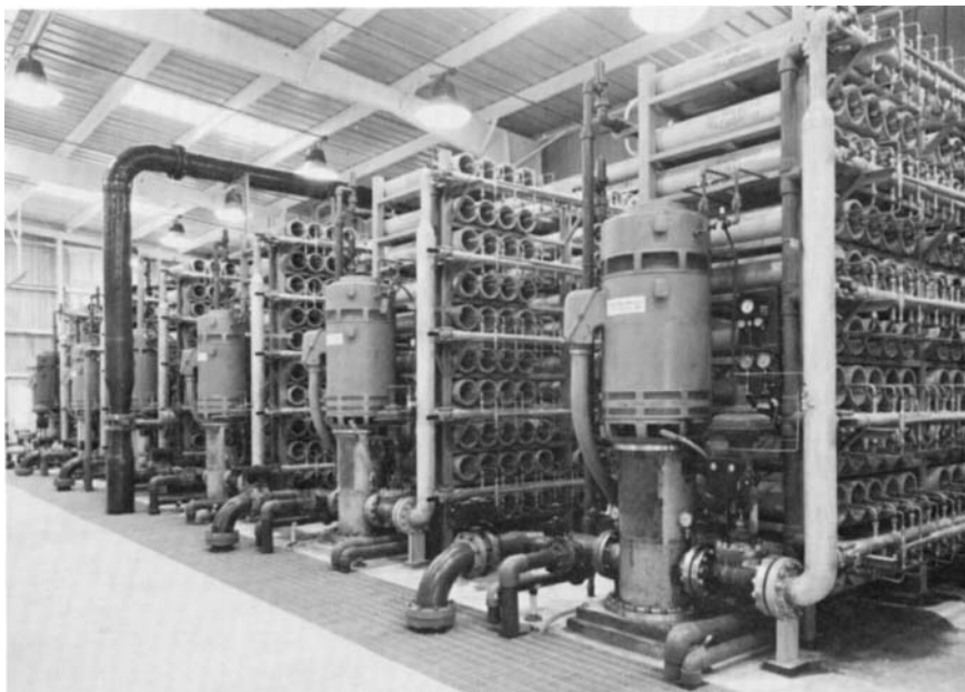
FIG. 15.15 At Key West, Fla., six banks of permeators process seawater with individual high-pressure pumps and controls to produce 0.5 mgd each of potable water. (Courtesy of Water Services of America and DuPont.)
