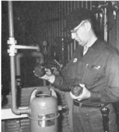
FIG. 37.2 Where there are multiple units to be treated, a simple feeder charged with briquetted chemical is often more practical than individual mechanical feeders.
