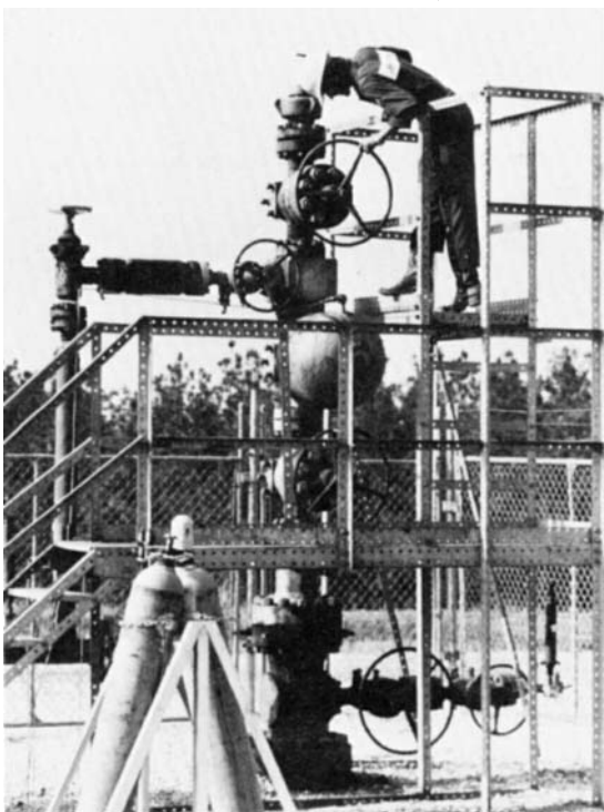
FIG. 43.5 This large "Christmas tree" is made up of 4-in valves and fittings designed for 10,000 lb/in 2 working pressure. (Courtesy of McEvoy Oilfield Equipment Company.)
