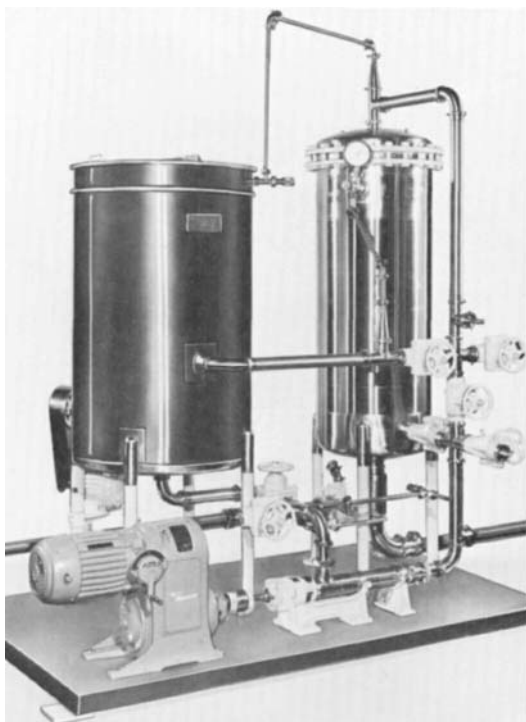
FIG. 28.3 A filter installation typical of the food and beverage industry practices. Note the use of special stainless-steel piping and fittings. (Courtesy of Cross-Reynolds Engineering Company, Inc.)
