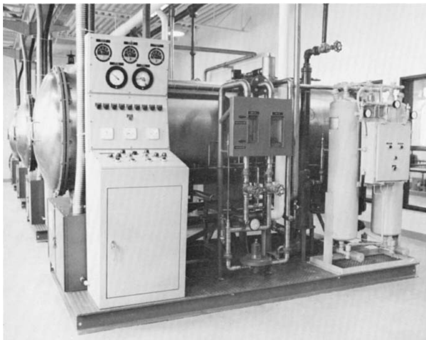
FIG. 22.10 A battery of three 110 lb/day (49 kg/day) ozonators installed in a municipal plant. These produce \text{O}_3 from air. (Courtesy of Infilco Degremont, Inc.)
