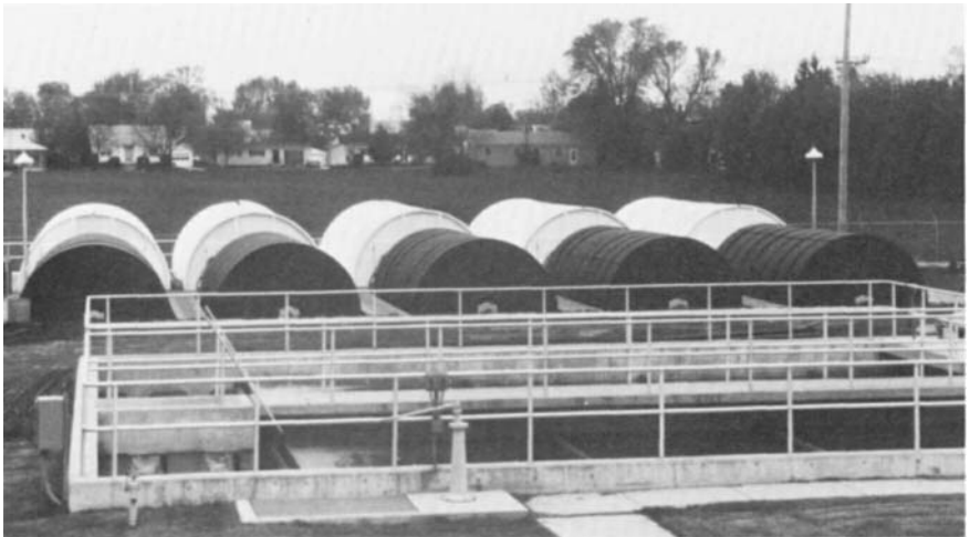
FIG. 23.17 In this 1.0-mgd sewage treatment plant, biological treatment takes place on these assemblies of disks mounted in basins through which pretreated sewage is flowing. A growth of biological gel develops on the rotating disks, providing the mechanism for digestion of organic wastes. Units are covered for odor control and to optimize temperature during winter operation. (Courtesy of Walker Process Corporation.)
