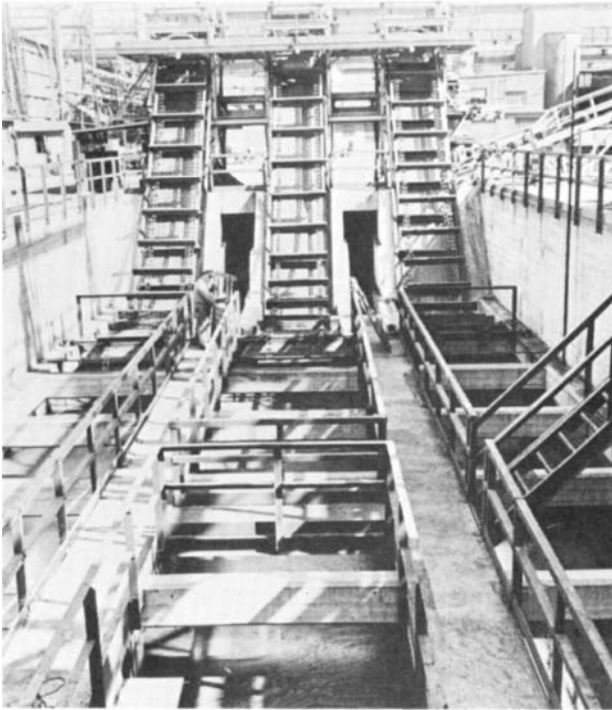
FIG. 9.20 Steel mill scale pit, provided with oil skimmer and sludge collector. (Courtesy of FMC Corporation.)
