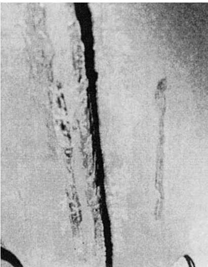
Figure 3-47. Damage to Valve Body Guide Ribs Resulting from Attempted Closure of Wedge Gate Valve with Rotated Wedge Jammed in Valve Body, Size DN 300 (NPS 12) Class 150. (Courtesy of David Mair.)
