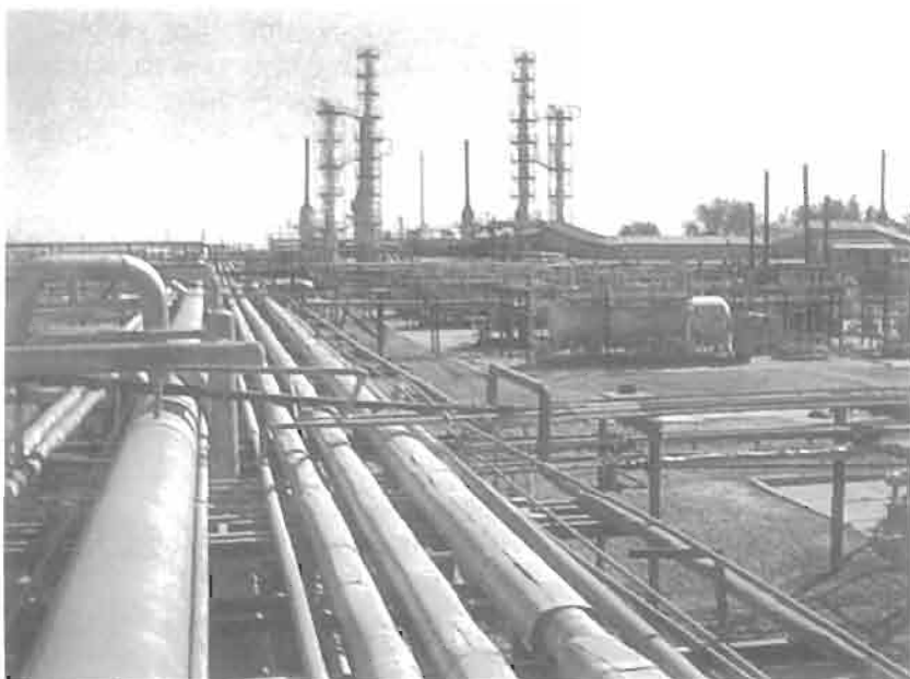
Figure 17. Gas processing plant operations.
