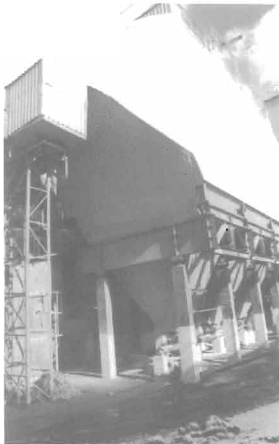
Figure 9 . New ESP installation servicing blast furnaces at a steel mill.
