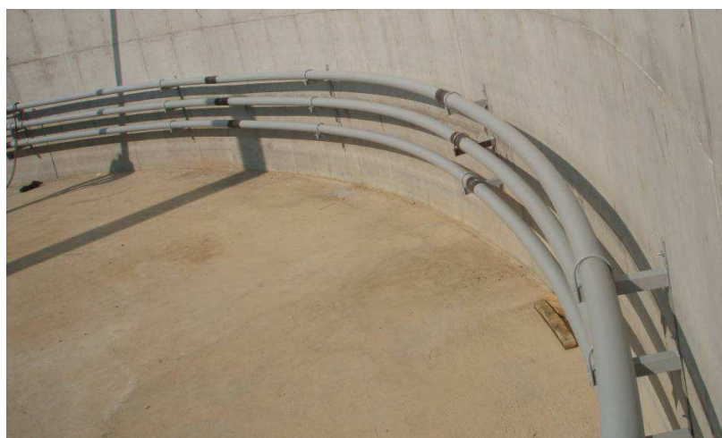
Figure 7.17 Heating pipes, installed inside the digester (AGRINZ 2008)
