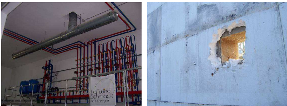
Figure 7.16 Heating system of a biogas plant ( left ) and insulation of a concrete digester, under construction ( right ) (RUTZ 2008)
