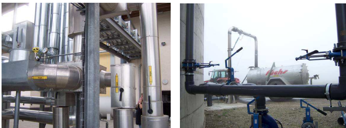
Figure 7.15 Insulated gas pipelines -left; Pipelines for digestate handling -right (RUTZ 2008)
