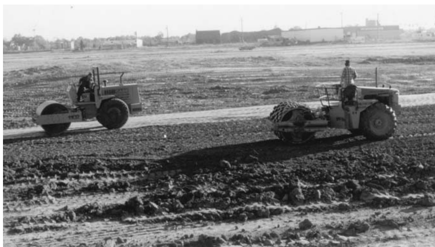
FIGURE 39.17 Vibratory and sheepsfoot rollers. (Photo Credit: Frost)
