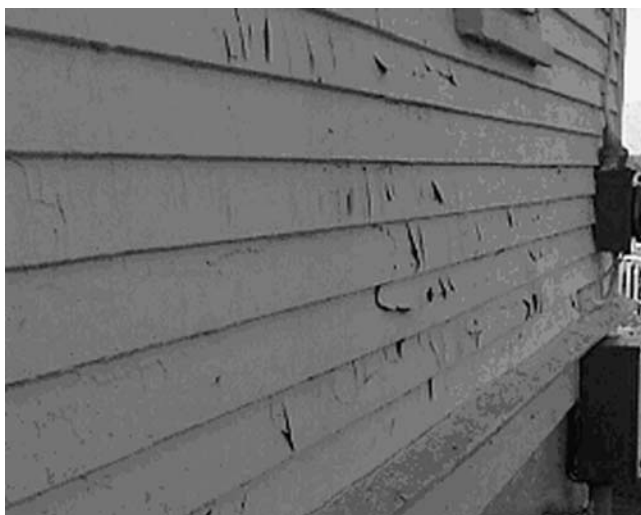
FIGURE 19.2 Lead-based paint peeling from a structure.
