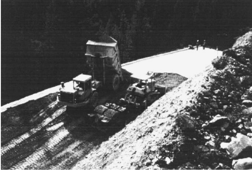
FIGURE 27.6 Placement of a high-strength nonwoven geotextile to perform a dual function of reinforcement and in-plane drainage in a reinforced slope.
