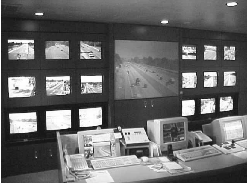
FIGURE 18.11 Traffic management center operation (courtesy ADA County High District, Boise, Idaho).
