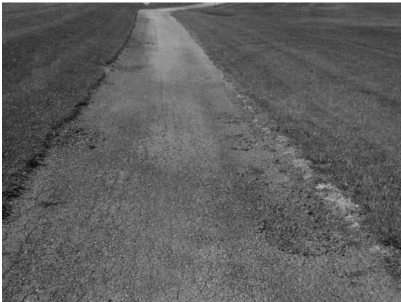
FIGURE 22.15 Rutting from maintenance vehicles on a shared-use path with substandard paving structure.
