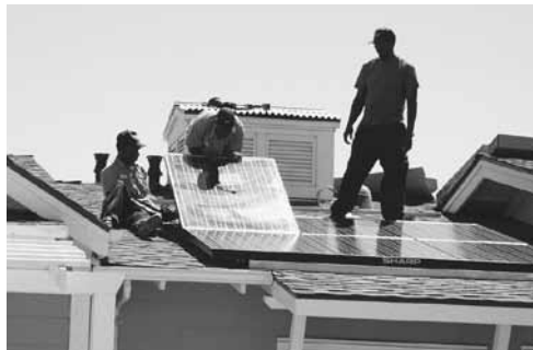
1.5 kW photovoltaic panel per house, a tight envelope, and shared community resources make for very low energy bills.
