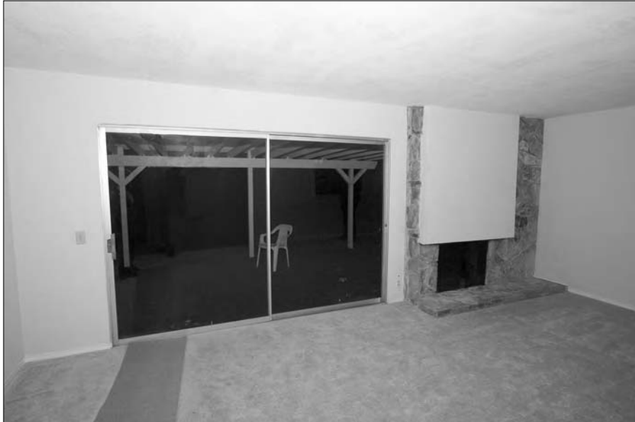
Figure 17-3: This old patio door looks weathered.
