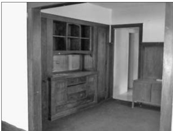
Figure 2-3: Before, 80 years of hard living takes an obvious toll.
