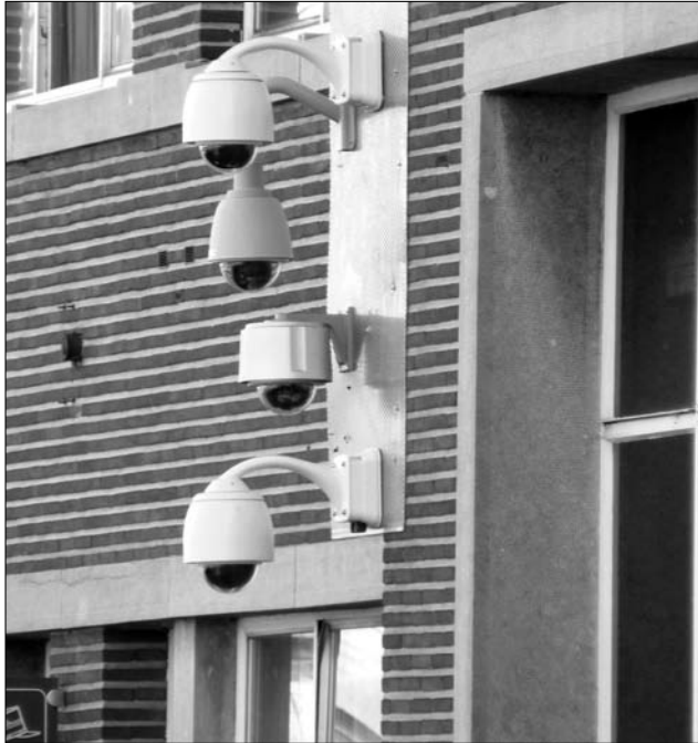
Figure 6-1: Surveillance cameras on the exterior of a building.
