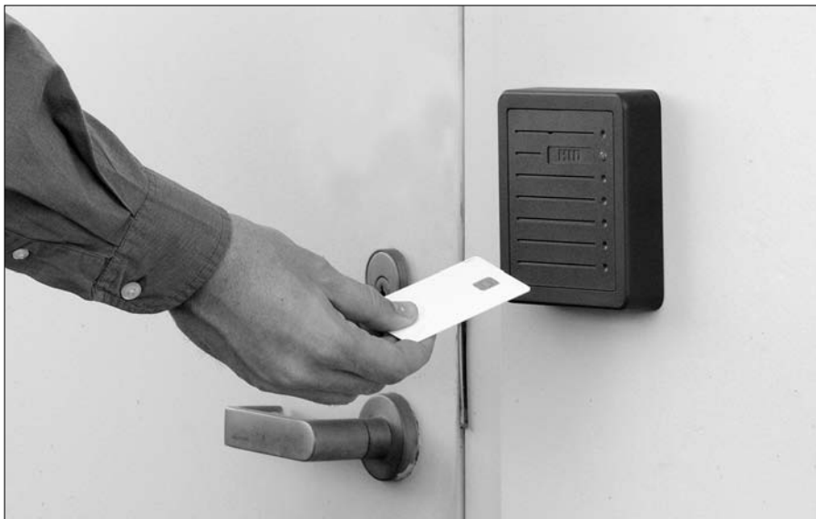
Figure 6-3: A contact-less proximity card reader permits users to enter a secure room or facility.
