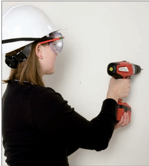
Figure 3-2: Drill your holes perpendicular to a wall by starting off at the right height.
