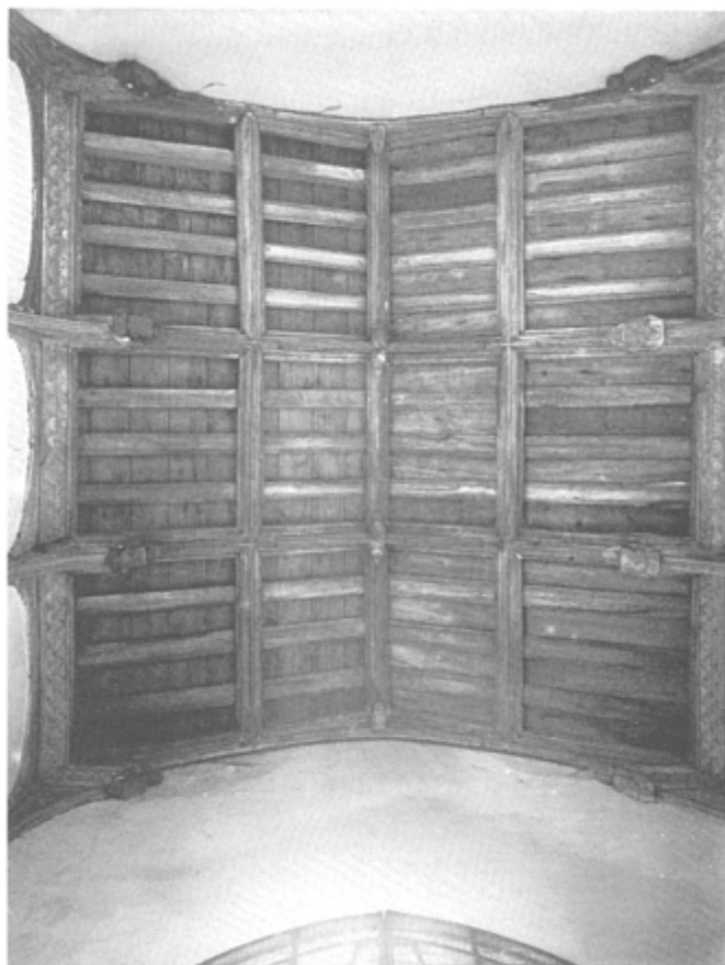
91 The porch roof at Swaffham Church, financed by William and Anne Coo who 'did make the Roffe of the porche'; fifteenth-century (R.C.H.M.)
