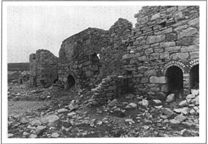
Plate 56 The derelict remains of Brunton calciners at Levant mine in Cornwall, once used for the production of arsenic on many tin mines. The consolidation of such structures has to encompass decontamination procedures.
