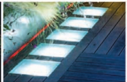
LED lighting should be installed by a professional.
