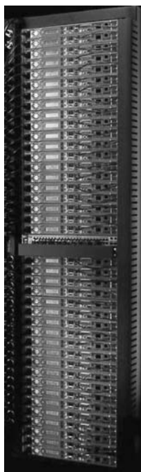
Figure 6.19 The TB-80 VME rack from Capricorn Systems used by the Internet Archive. All cables, switches, and displays are accessible from the front side, and so the back side is only used for airflow. This allows two racks to be placed back-to-back, which reduces the floor space demands in machine rooms.
