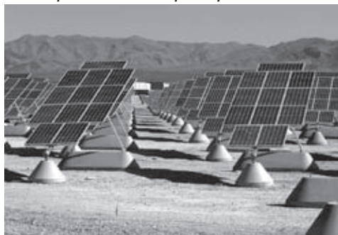
A photovoltaic solar power plant in Nevada
