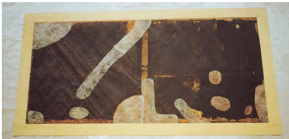
Figure 23.63 The finished repairs complete with the strip lining. Note the distortion caused by the painted pattern in the left half.
