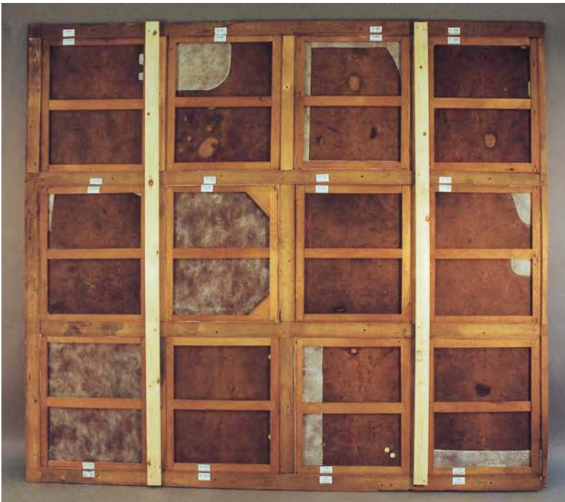
Figure 23.86 The back of a completed section of panelling showing two full linings and smaller repairs.
