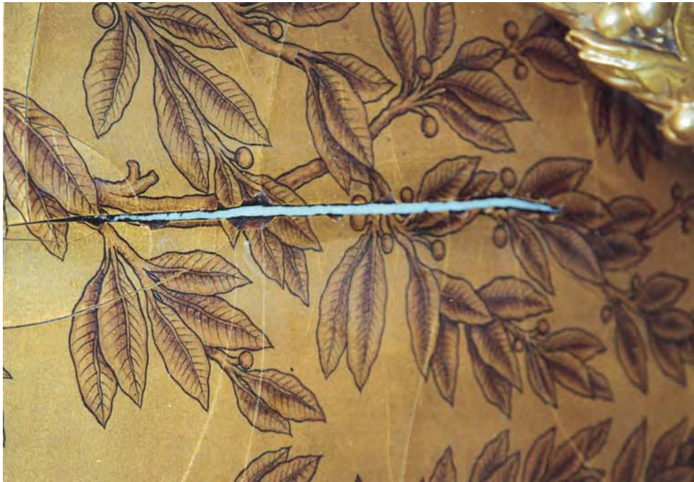
Figure 23.1 Major split in roof and cracks in the paint surface. The sailcloth has been inserted.
