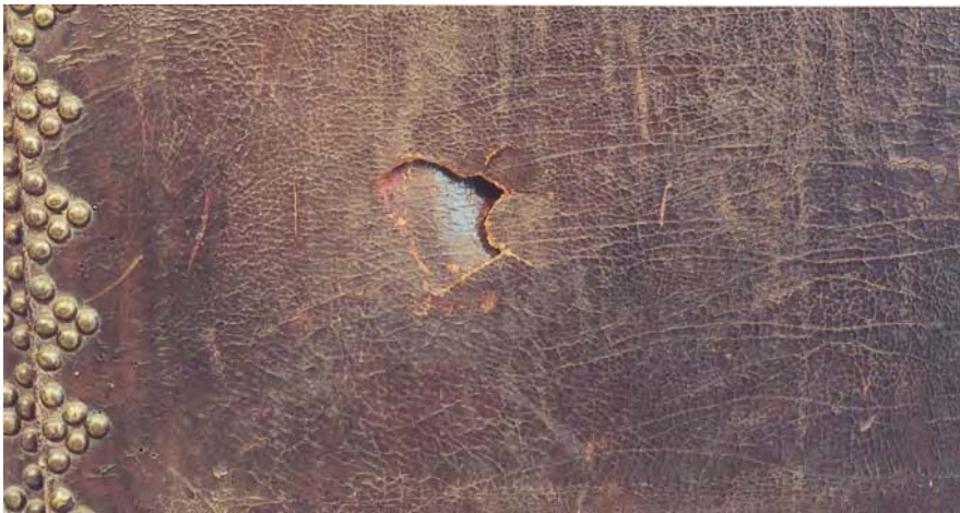
Figure 23.23 Damage before repair using low pressure suction box.
