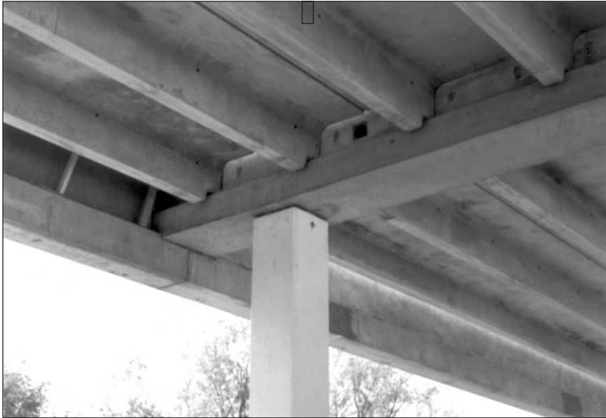
Figure 9.2: Beam-to-column head connections. A bearing pad and grouted dowels are also present.
