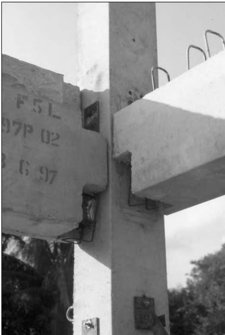
Figure 9.1: Beam-to-column face connections. Asymmetrically loaded beams require couple connections to prevent beam twisting.
