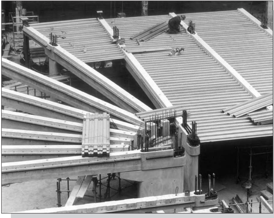
Figure 1.12: Mixed cast in situ and precast concrete, with composite steel decking floors (courtesy Trent Concrete, UK).
