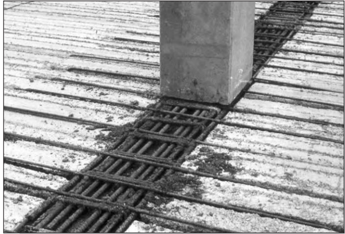
Figure 5.23: Reinforced cast in situ concrete forms a composite beam with hogging resistance and continuity.
