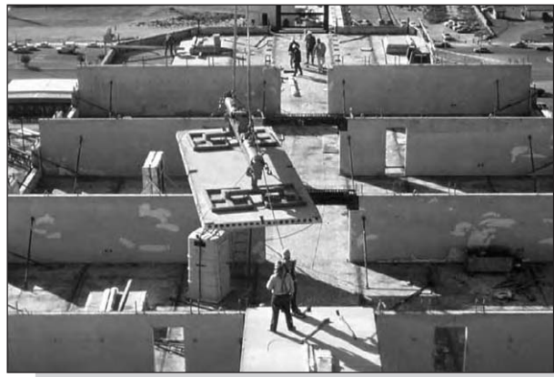
Figure 3.3: Wall frame with 3.6 m wide hollow core floors (courtesy A. Curd and Partners, USA).
