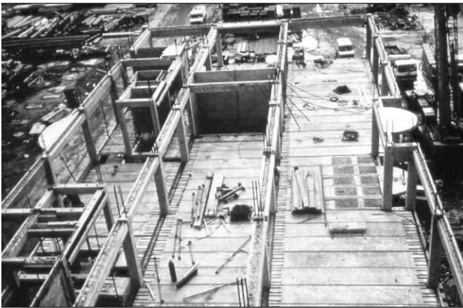
Figure 7.1: Precast concrete hollow core floor diaphragm in multi-storey construction (courtesy Reinforced Concrete Council, UK).
