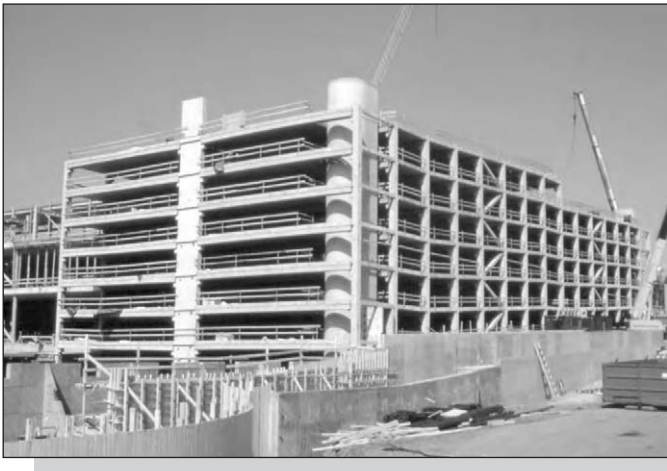
Figure 1.5: Precast concrete skeletal structure – The 'Green Apple' retail centre near Helsinki, Finland.
