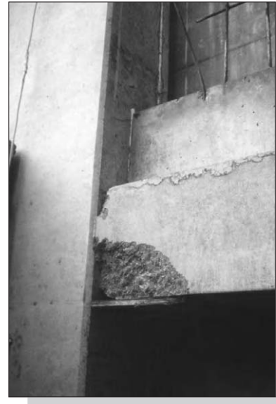
Figure 9.5: Damage to beam end due to lack of fit and/or spurious hogging moments.
