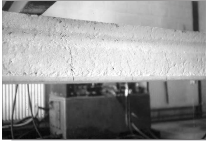
Figure 4.14: Flexural cracking in hollow core slab.
