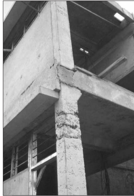
Figure 2.2: Compaction problems in a precast concrete column.
