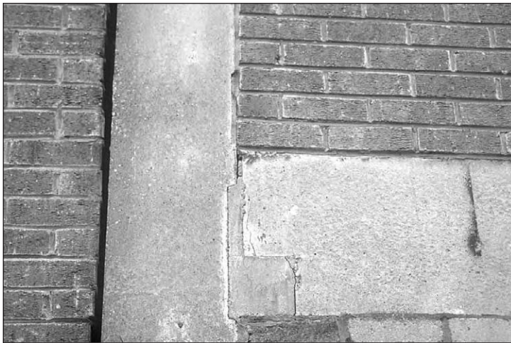
Figure 9.24: Shrinkage and other movement cracks around the edges of grouted up recesses.
