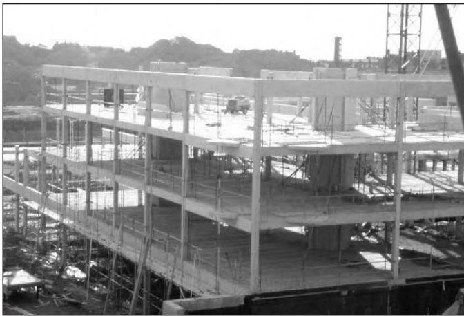
Figure 3.1: Precast skeletal structure showing large unobstructed spaces for the benefit of both the construction workers and client.
