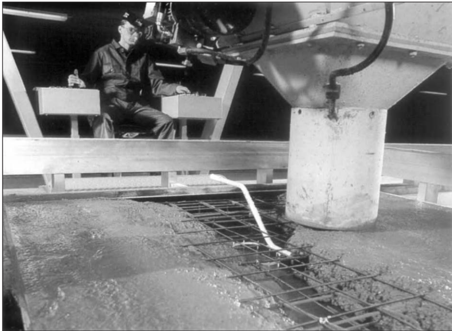
Figure 2.1: Precise delivery of concrete to the mould (courtesy Tammer Elementti Oy, Finland).
