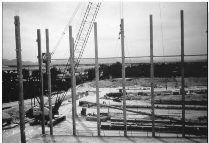
Figure 6.3: 25 m long single piece columns at MGM car park, Las Vegas (courtesy Andrew T Curd & Partners, USA).
