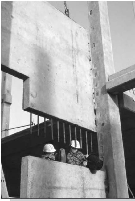
Figure 6.32: Horizontal interface shear reinforcement and vertical welded joints in an infill wall.
