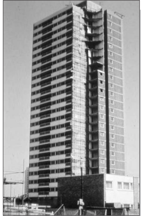
Figure 10.1: Progressive collapse of precast wall frame at Ronan Point.
