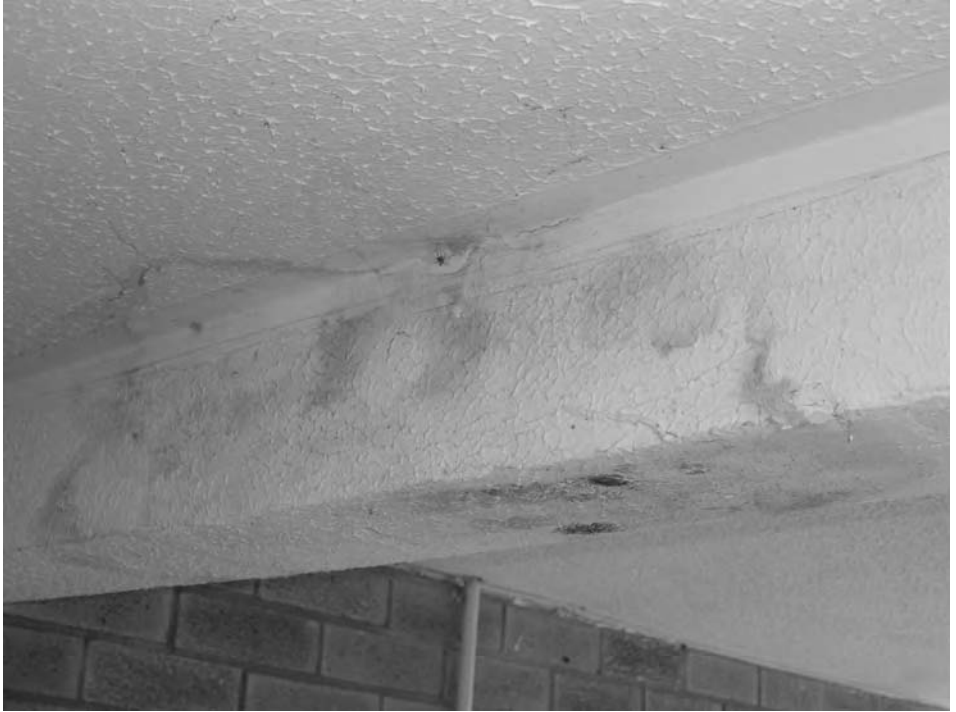
Figure 7.2 Mould growth on steel lintel in a garage
