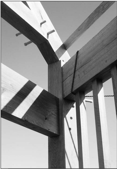
Figure 13.40: Traditional timber frame construction. Wooden plugs are used for fixing. Source: Gaia Lista, 1992
