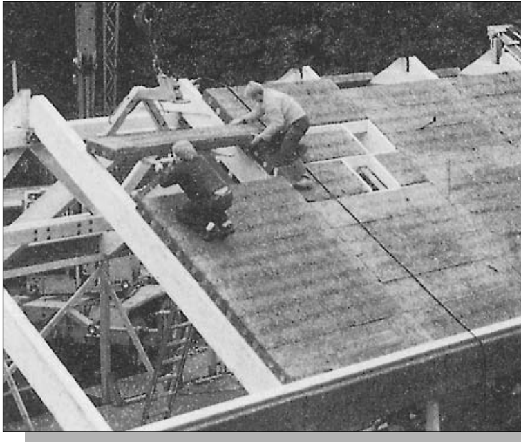
Figure 14.13: Woodwool slabs reinforced with round rods combine high thermal insulation values with structural integrity.
