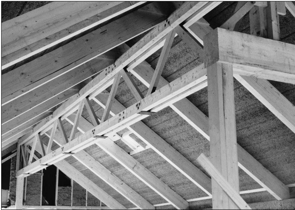
Figure 13.31: A lattice I-beam in a bakery. All joints are fixed by bolting; no glue is used. Source: Gaia Lista, 1990
