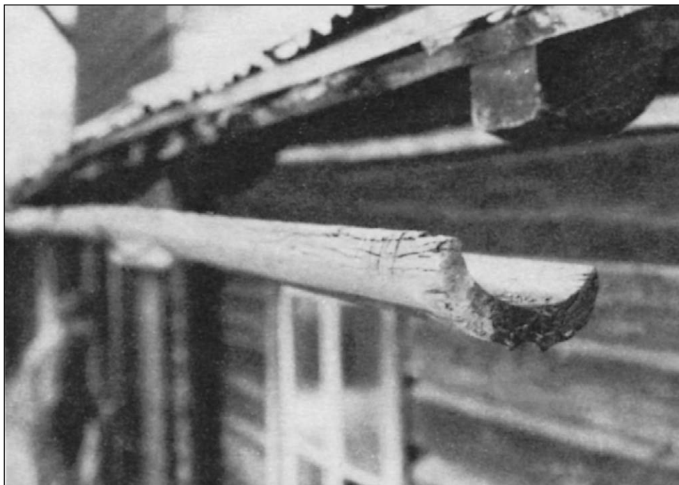
Figure 14.5: A wooden gutter, well worn after decades of service.
