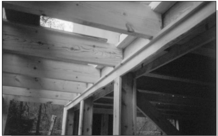
Figure 13.34: A structure designed for re-use. The structure is made of prefabricated standard monomaterial components, timber and concrete, which can easily be dismantled and re-used. Source: Gaia Lista, 1995
