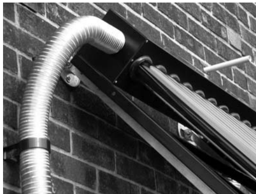
Well-insulated pipework and warm water recirculation is a new alternative to antifreeze in solar water heating installations (Reproduced with permission from Powertech Solar)
