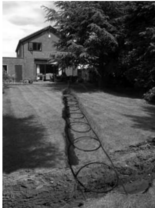
Horizontal closed loop system with horizontal 'Slinky' layout (Reproduced with permission from ICE Energy Heat Pumps)
