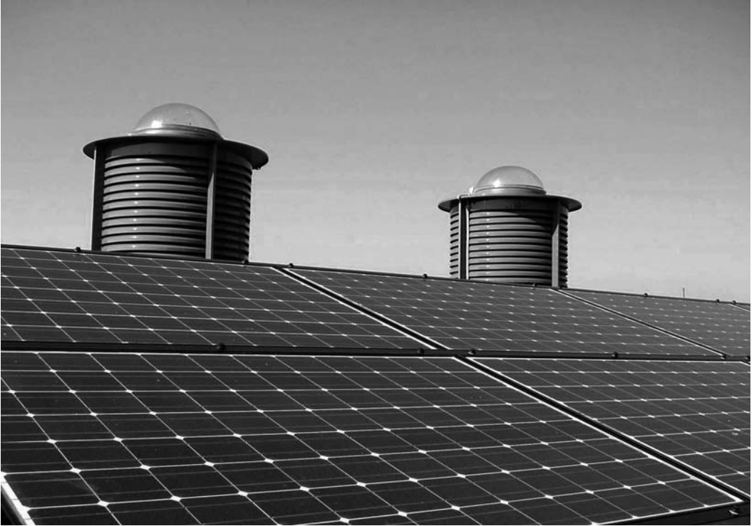
This roof features solar PV, windcatchers and lightpipes (Reproduced with permission from Monodraught)
