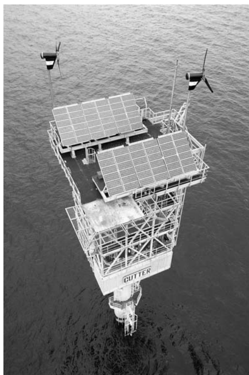
Wind turbines and solar PV are an effective combination on this offshore installation (Reproduced by permission from Eagle Power)
