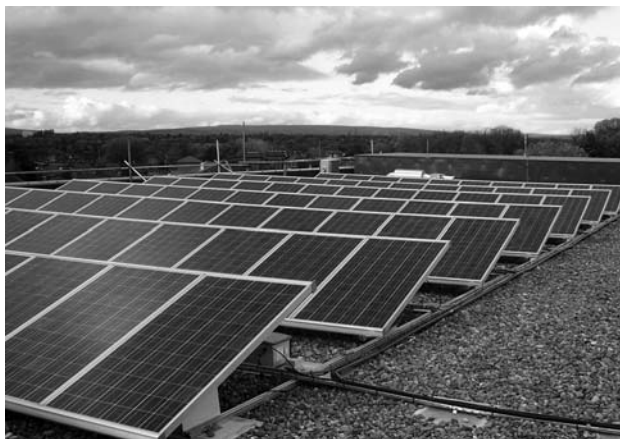
Roof-mounted modules supplement the PV façade (Reproduced with permission from Solarcentury.com)
