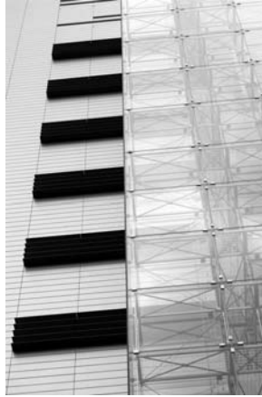
Cooling air intakes are blended into the façade (Reproduced with permission from Mott MacDonald)
