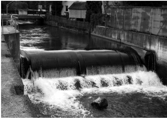
This Austrian example is typical of the existing weirs that could be utilised for small hydro (Reproduced with permission from European Small Hydro Association/KO)
