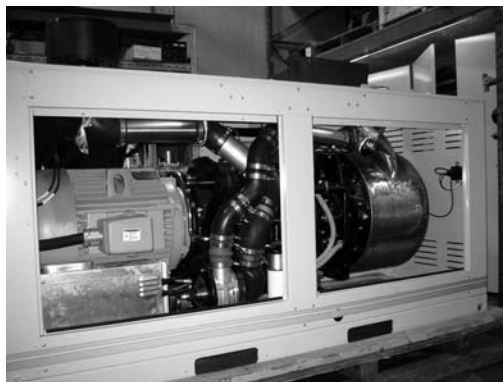
This Stirling engine generator set by STM Power produces 55 kW and can run on biofuels and biogas (Reproduced with permission from Wtshymanski)
