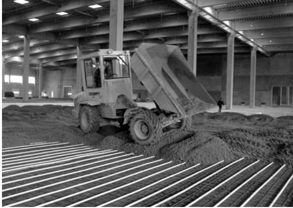
Underfloor heating is suitable for the largest buildings (Reproduced with permission from Nu-Heat UK)
