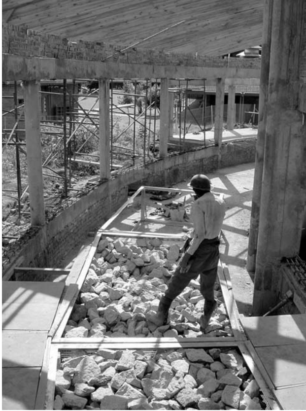
Rock bins using large aggregate have proved very effective (Reproduced with permission from Arup – Mike Rainbow)
