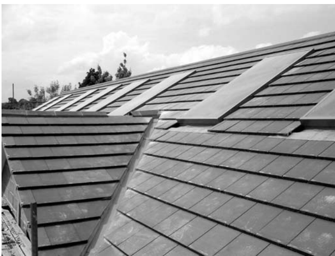
Roof-mounted thermosyphoning air panels can be unobtrusive (Reproduced with permission from Nuairé)
