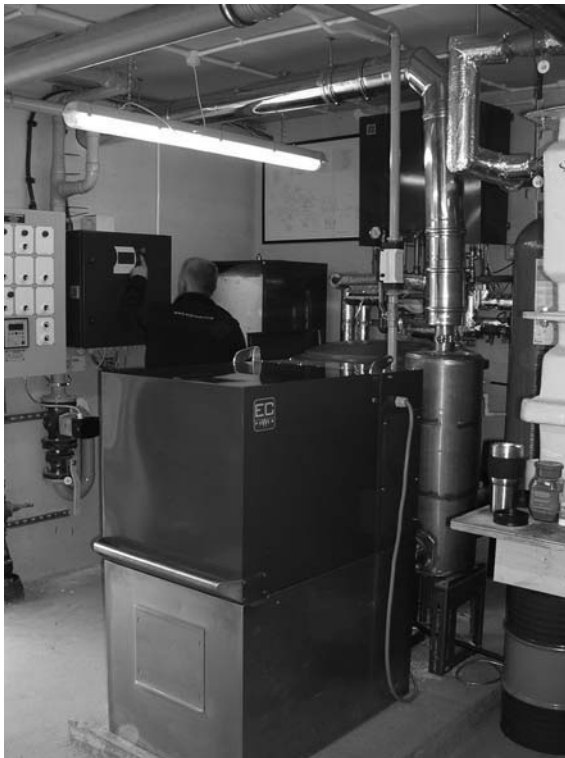
Natural gas fuelled CHP, like this 15kW installation from EC Power, is a well-developed technology (Reproduced with permission from EC Power)
