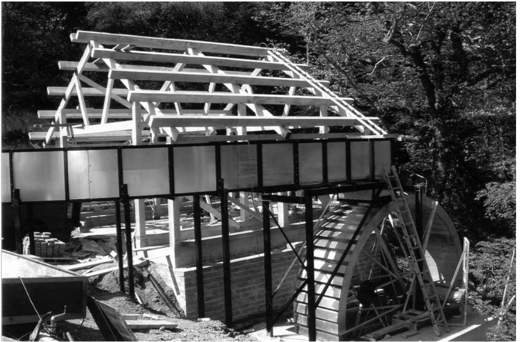
The visitor centre and waterwheel during construction (Reproduced with permission from Tony Robson consultant)
