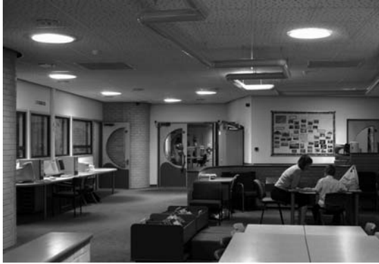
Intelligent use of light pipes can slash lighting costs (Courtesy of Monodraught)
