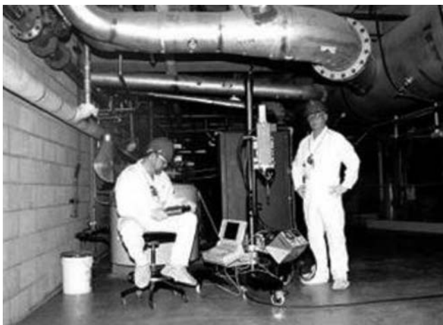
FIGURE 3C.4 A large overhead duct is measured from below with a collimated Ge detector.
