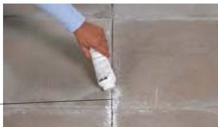
Sprinkle ant powder into any cracks where ants appear
