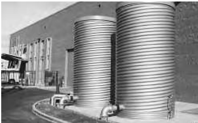
At the new Tacoma, WA, police facility designed by TCF Architecture, two 4,800-gallon tanks collect rainwater and recycle it for toilet flushing.
