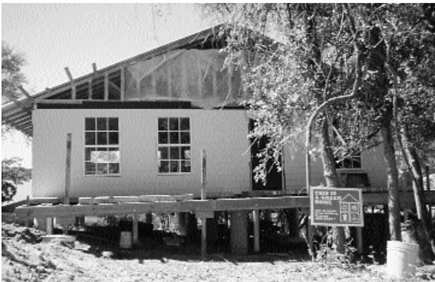
The Green Builder program in Austin, Texas, has done much to educate and promote environmentally friendly building. Shown here is a green-builder certified home under construction in east Austin.
